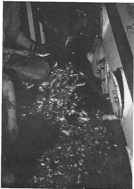
Condensator B.B. turbo-generator.
